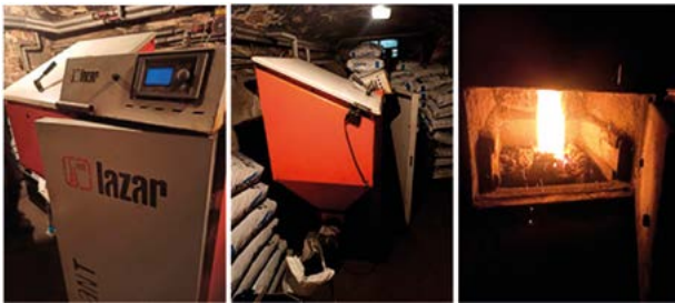
Figure 4. View of the boiler no. 4 Source: Own elaboration.
