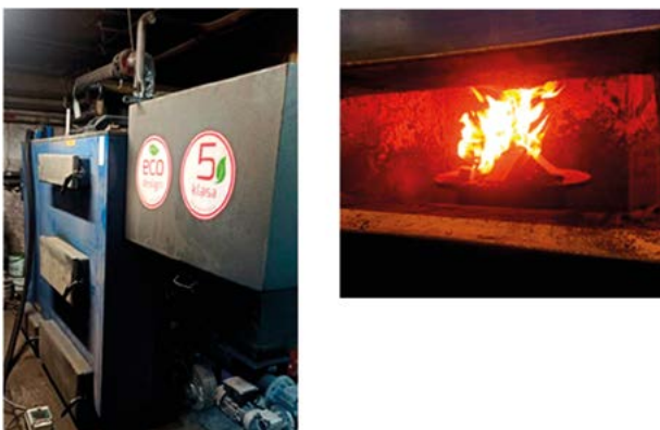
Figure 5. View of the boiler no. 5 Source: Own elaboration.
