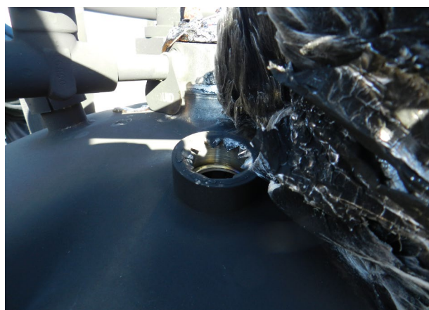
Figure 5. Broken vacuum fuse
