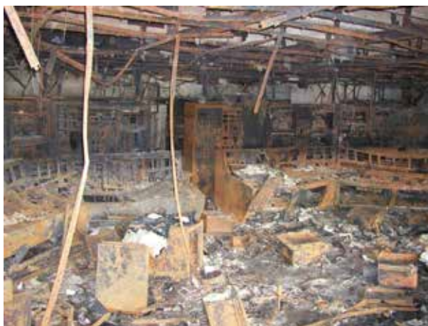
Rycina 11. Skutki pożaru w nastawni w elektrowni Figure 11. The effects of a fire in the power plant's control room
