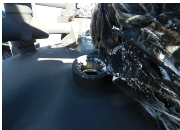
Figure 5. Broken vacuum fuse
